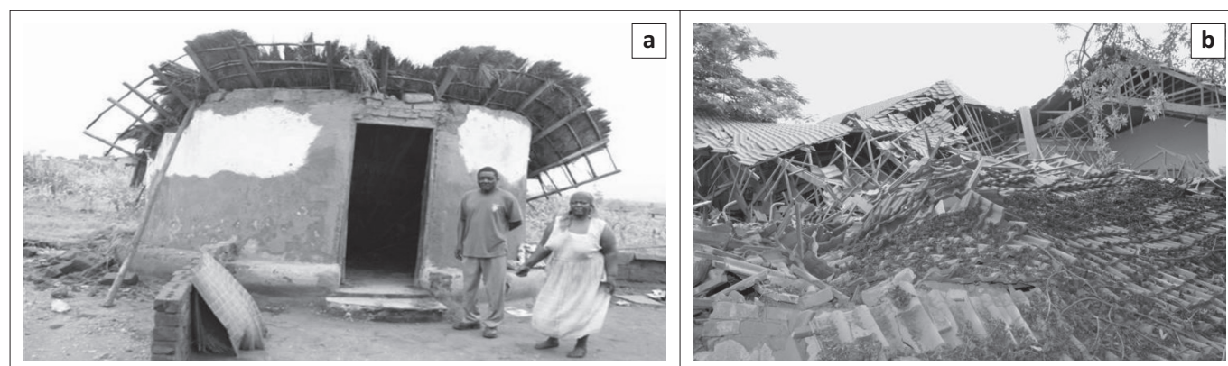
Source: Vhembe District Disaster Management Center flood disaster report 2011 FIGURE 6: Houses crumbled by flood at (a) Tshilungwi and (b) Maniini.
