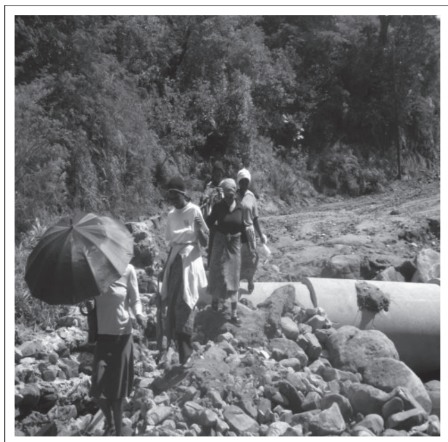
Source: Vhembe District Disaster Management Center flood disaster report 2011 FIGURE 5: Damage to road and culvert (Road D3688) – Tshilungwi Village.
