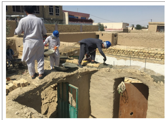
FIGURE 8: Additional brick works on the top of the existing wall and making connection using steel bars.
